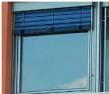
External blinds – above plaster system
